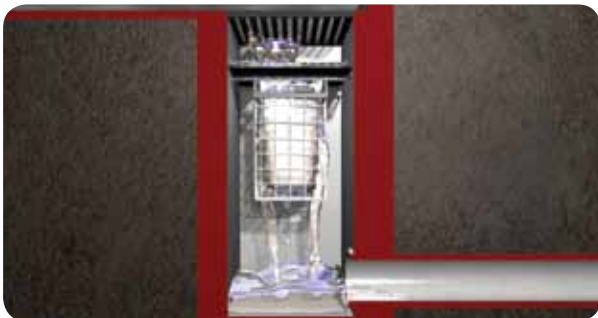
Screening EnviroPod – located with each gully pit
